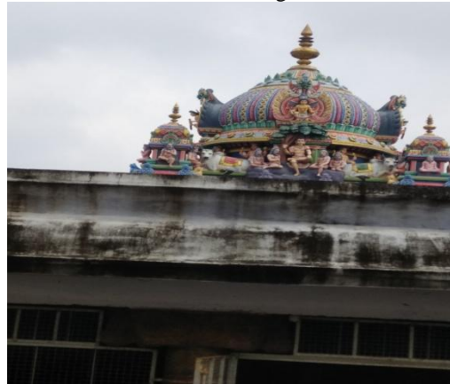
Figure 4: Discoloration of stone heritage at AIYARAAPAR temple
