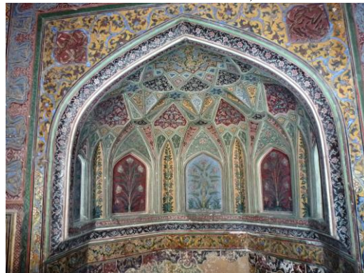
[Plate-4b.] Wazir Khan Mosque, Lahore Depicting the Fresco Painting deteriorating at the base.
